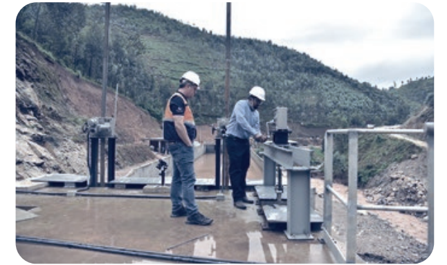
March 2022 – Commissioning of Omnihydro powerplant in Rwanda
